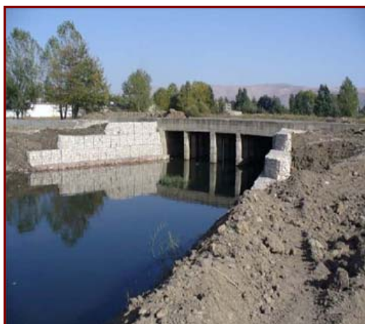
An example of a rehabilitated canal from AVSI's interventions along the Litani River
